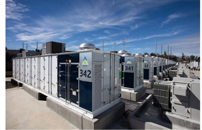
AES 30 MW / 120 MWh ESS, Escondido, CA Peaker replacement
