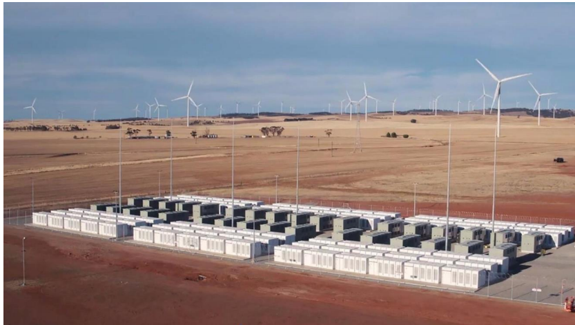
Tesla 100 MW / 129 MWh ESS Australia - Grid stability
