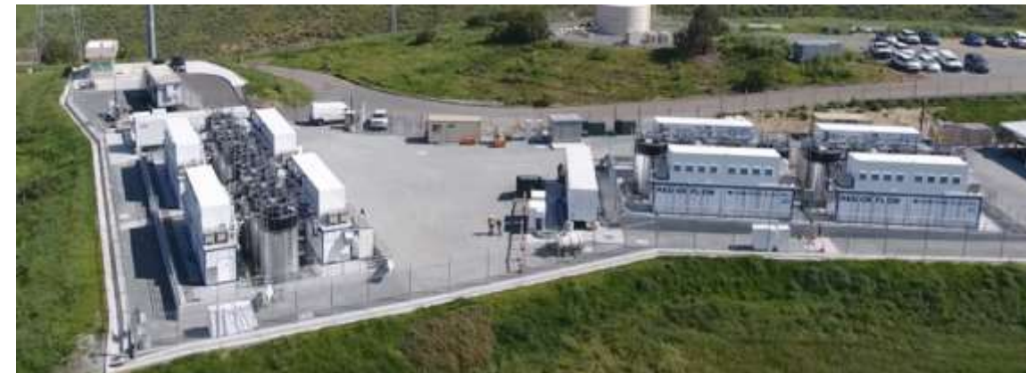
Sumitomo 2MW/8MWhr vanadium Redox Flow Battery system in San Diego, CA
