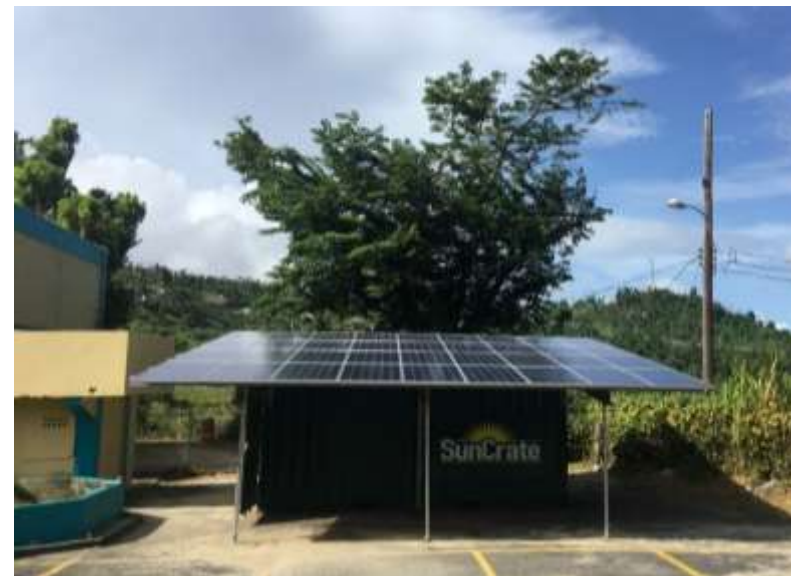
Earlier microgrid: Solar crate in Puerto Rico, August 2018
