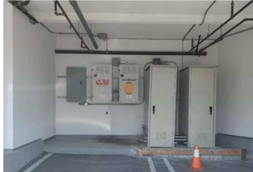
AC Concentration Panel, (2) 30kW Inverters, and 60 kW/110kWh Battery Energy Storage System
