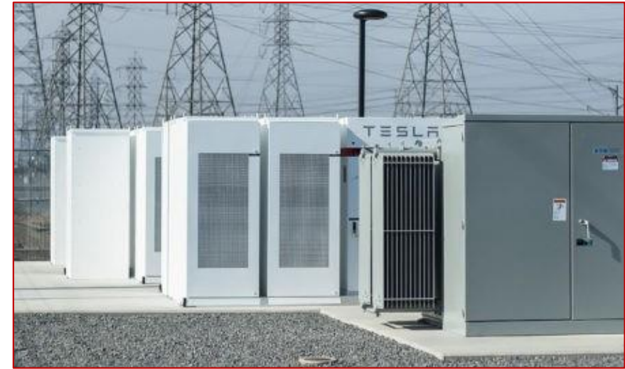
SCE/Tesla 20MW - 80MWh Mira Loma Battery Facility
