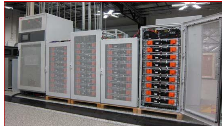
SCE Tehachapi Plant, 8MW–32MWh
