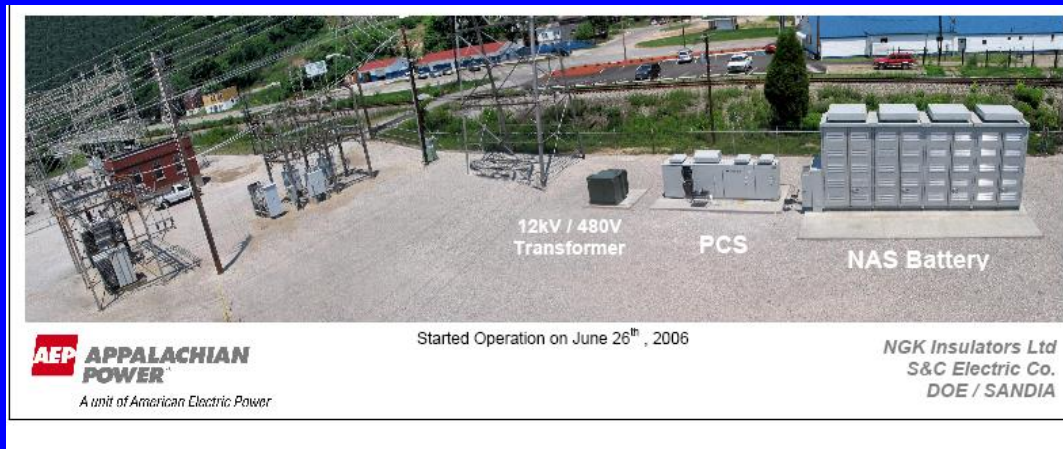
Charleston, WV Appalachian Power Substation
