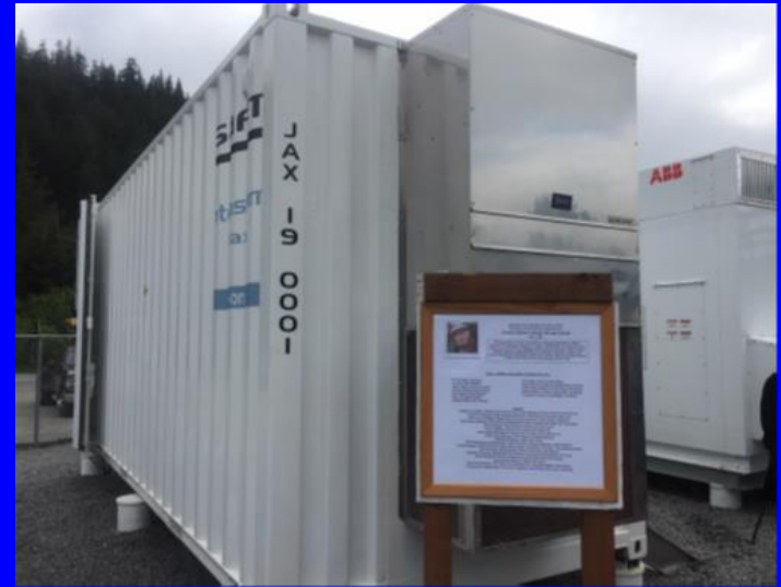
1 MW / 1 hr Li-ion Storage
