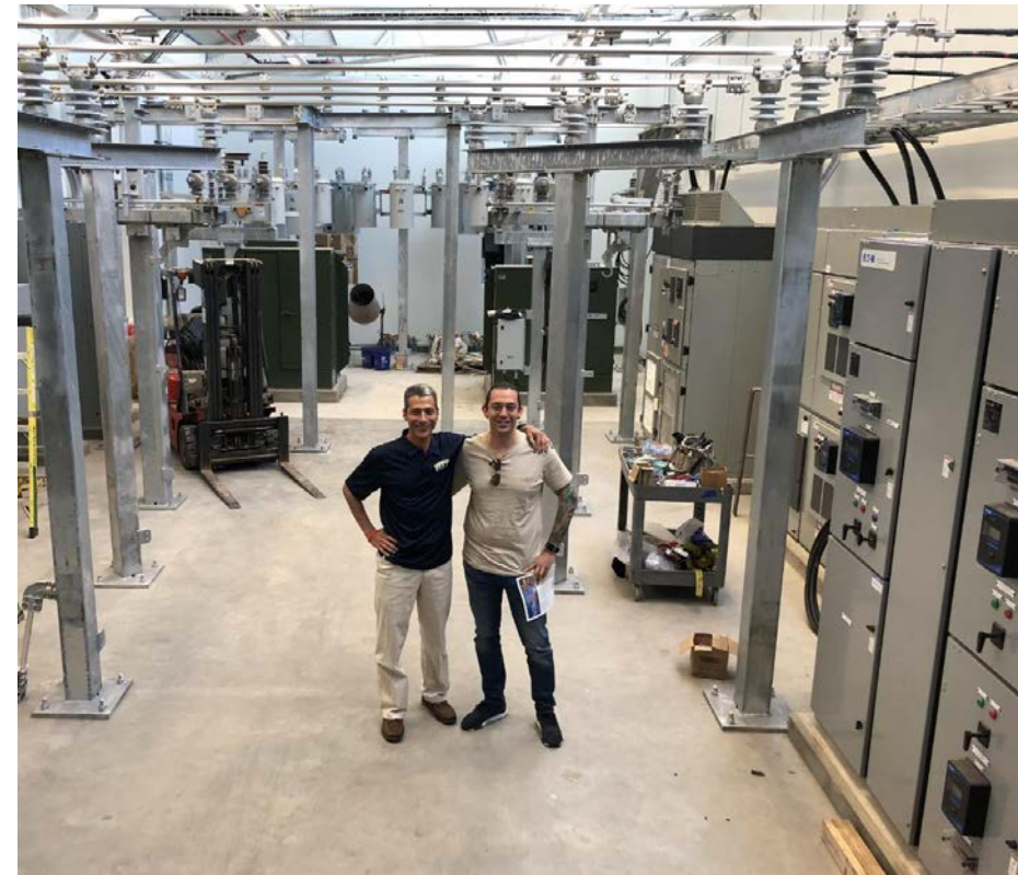
13.8 kV / 4.16kV portion of High Voltage Laboratory at the University of Pittsburgh GRID Institute
