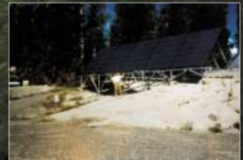
△ Solarex provided this 7kW remote system for Southern California Edison at Big Creek, Mammoth Mountain. Shown is one of the arrays featuring 60 MSX-60 modules. [Photo courtesy Solarex]
