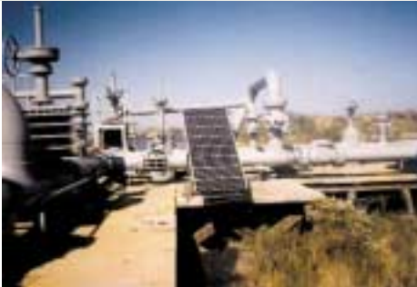
△ Remote telemetry for monitoring oil, gas and water pipelines is a common application for photovoltaics. Kyocera Solar, Inc. installed this monitoring system. [Photo courtesy Kyocera Solar, Inc.]
