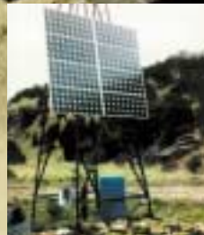
◁ This U.S. Army installation at Ft. Carson, Colorado, takes advantage of photovoltaics for a water pumping project. [Photo courtesy U.S. Army]
