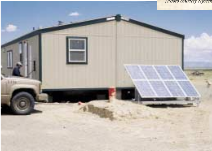
△ Kyocera Solar, Inc. provided 600W skid-mounted PV systems for 100 homes on the Navajo Reservation. The installations were purchased and installed by the Navajo Tribal Utility Authority (NTUA). [Photo courtesy Jimmie Daniels, NTUA]
