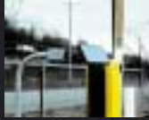
◁ An 18 watt Solarex panel provides power for a parking lot security system and light. [Photo courtesy Atlantic Solar Products]
