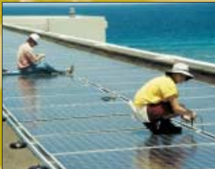
△ Mauna Lani Hotel and Bungalows, Kohala Coast, Hawaii. This unique 100kWp (75kWAC) solar electric tile system is believed to be the largest hotel PV system in the world. PowerLight Corporation, integrator, installed their commercial-scale PowerGuard system using ASE's PV modules, backed with insulating polystyrene foam. The project exemplifies the
