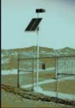
△ Yuma Proving Ground uses small PV arrays to provide security lights at vital locations. [Photo courtesy U.S. Army]
