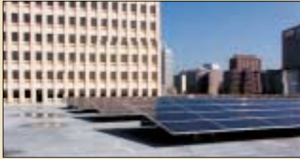
△ This large 20kW system was designed and installed on the Houston Health Science Center by Planergy, Inc. [Photo courtesy Planergy, Inc.]
