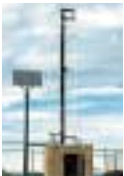
◁ Cellular repeaters are often very large or for other reasons are not always good candidates for photovoltaics. This installation by Solar Depot, however, serves an appropriate application of PV for this purpose. [Photo courtesy Solar Depot]
