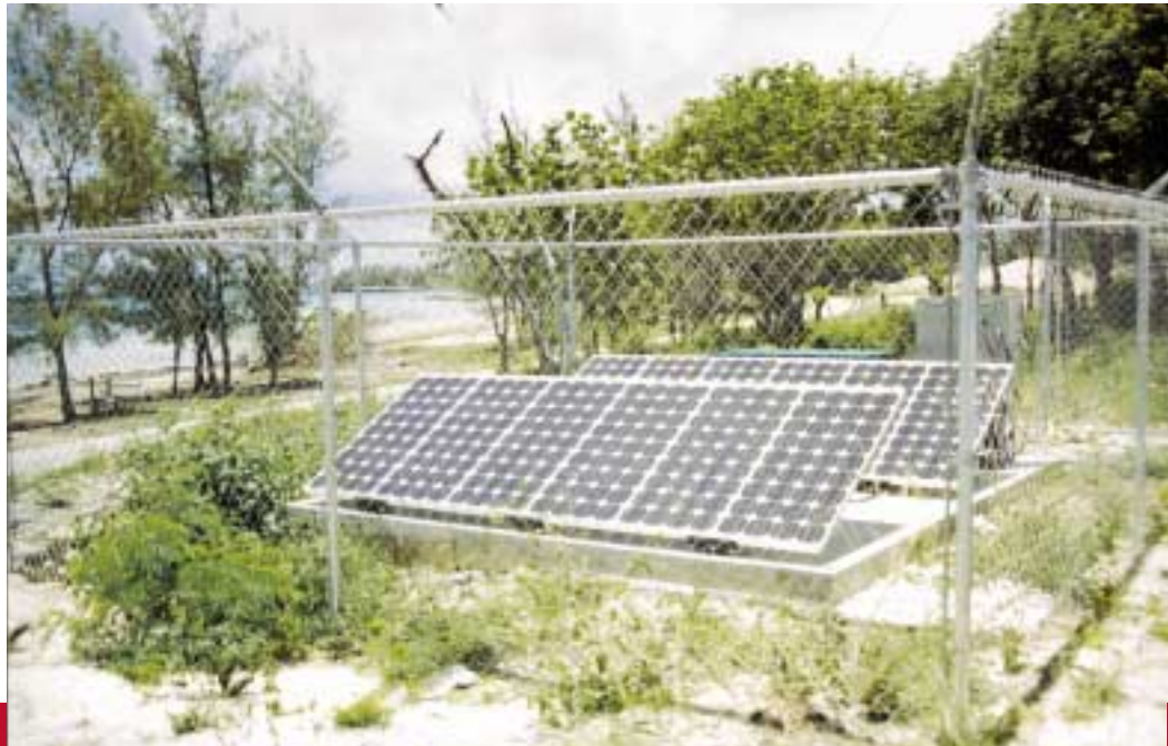
▽ On a lonely stretch of beach between two Florida cities, a cable TV operator discovers greatly increased customer service through the use of solar energy. This system is powered by a 900W SEPCO system, which contains 21kWhs of sealed Gel battery storage located at the far side of the array. [Photo courtesy Solar Electric Power Company – SEPCO]
