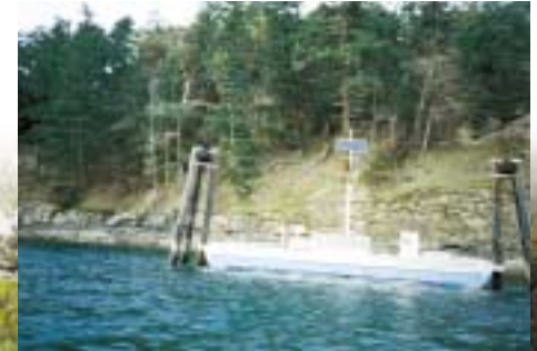
△ This small PV installation at the dock at Stuart Island, San Juan Islands, Washington, is sufficient to power an effluent dump station for boats that dock there. [Photo courtesy Sandia National Laboratories]
