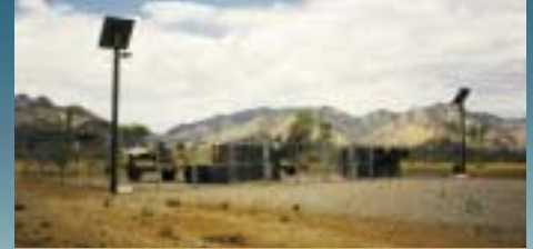
△ The military often uses photovoltaics to power remote facilities, such as this area lighting at a remote equipment storage facility at Fort Huachuca, Arizona. [Photo courtesy U.S. Army]
