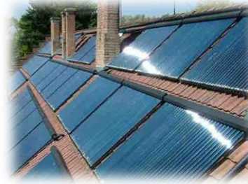
Solar Water Heating
