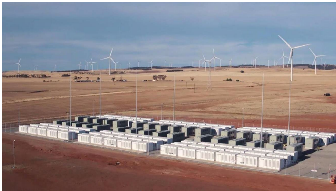
Tesla 100 MW / 129 MWh ESS Australia - Grid stability
