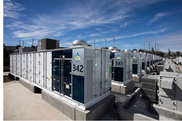
AES 30 MW / 120 MWh ESS, Escondido, CA Peaker replacement
