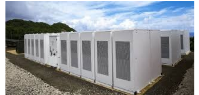
100 MWh BESS Plant - Tesla
