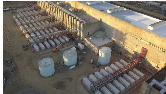
Vistra Energy, Moss Landing, Monterey, CA - 300 MW / 1200 MWh - Peaker Replacement, Grid Reliability
