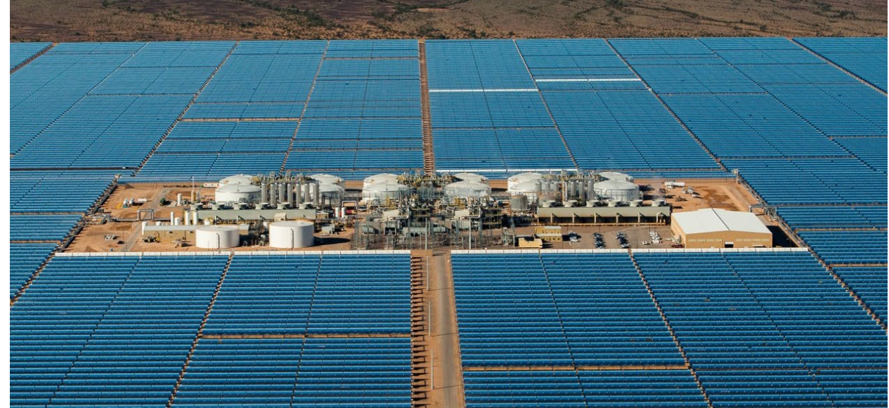
Solana Parabolic Trough Solar Project 1.5 GWh e storage in 6 pairs of hot and cold tanks.
