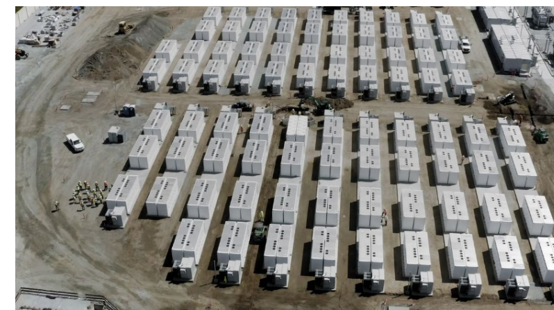
Tesla Megapacks, Moss Landing
