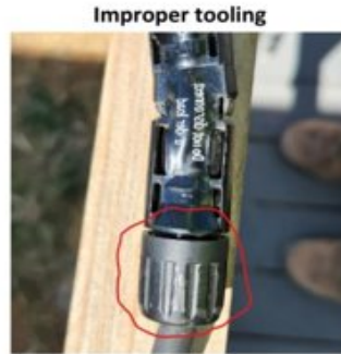
Evidence of improper tooling used for torquing
