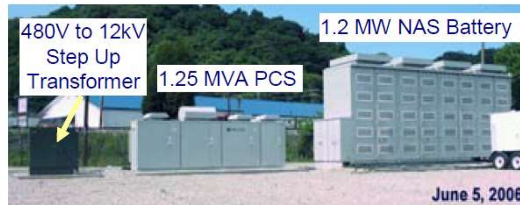
Figure 14 – Photographs of AEP's Chemical Substation before & after installation of 1.2 MW DESS in line with a 12kV feeder
