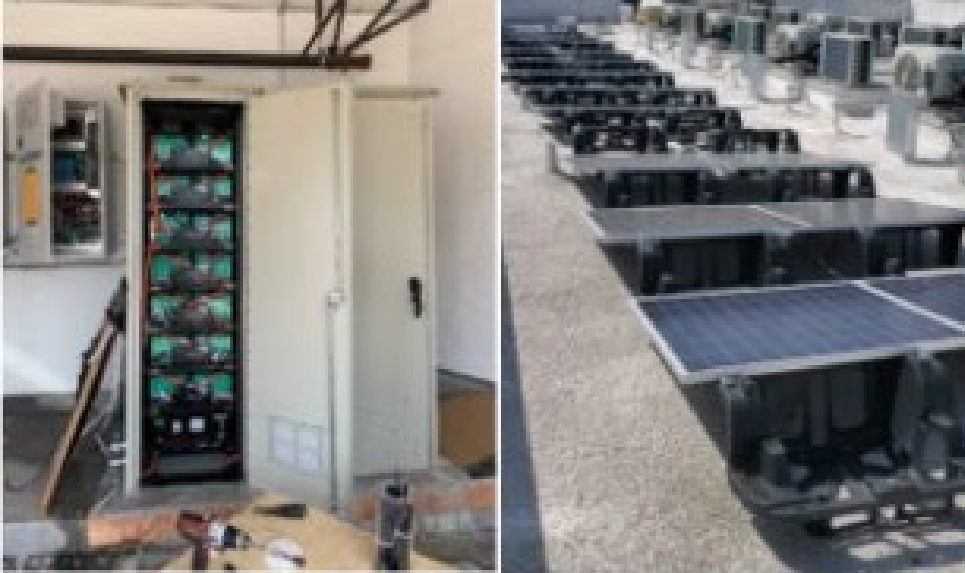
EnerPort L3060 Battery Installation
