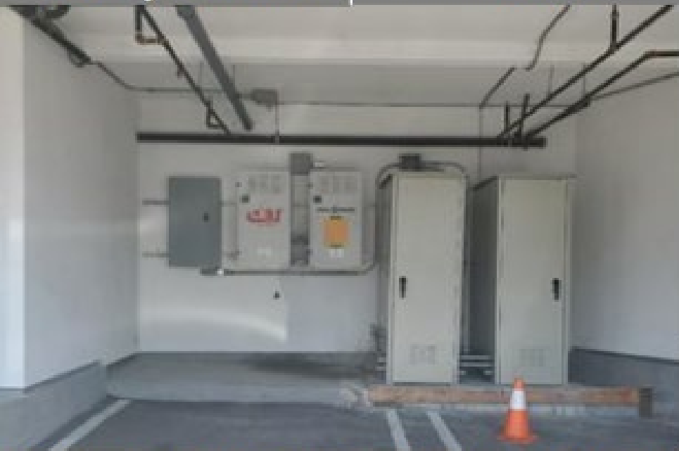
AC Concentration Panel, (2) 30kW Inverters, 60 kW/110kWh Battery Energy Storage System
