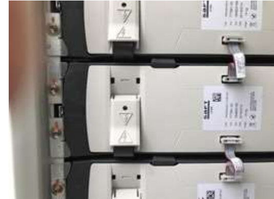
Typical module in a Rack
