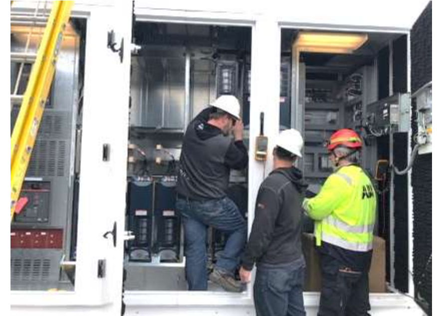
ABB Inverter line-up at Cordova
