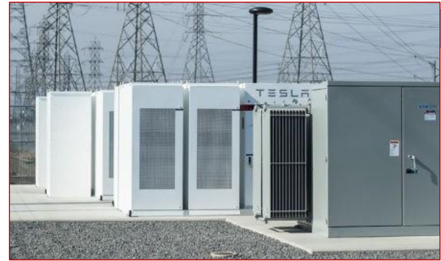
SCE/Tesla 20MW - 80MWh Mira Loma Battery Facility
