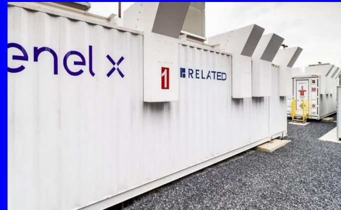
Li-ion batteries by ENEL-X
