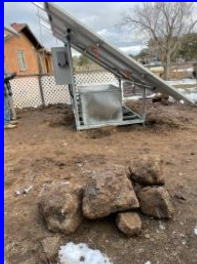
Native Renewables Navajo and Hopi Res, NM, AZ Off Grid Solar + Storage
