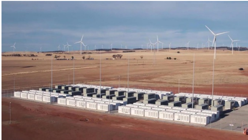
Tesla 100 MW / 129 MWh ESS Australia - Grid stability
