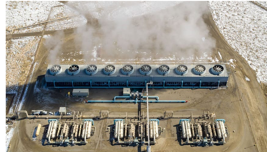
Fervo Energy's 3.5-megawatt enhanced geothermal plant in Nevada. (Google/Fervo)
