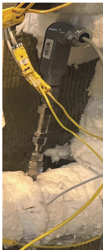
Figure 18. FEES sensor installed in industrial partner's flow loop
