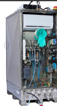
CA Pumped Loop
