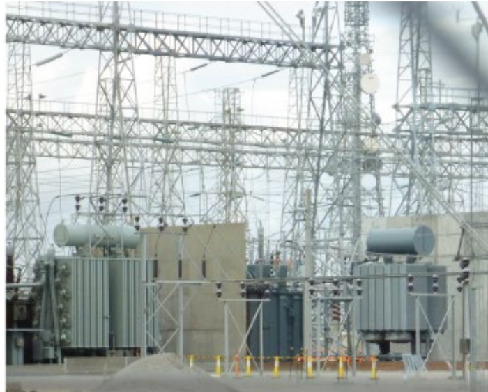
Two of five transformers in transmission substation, Melbourne, Australia
