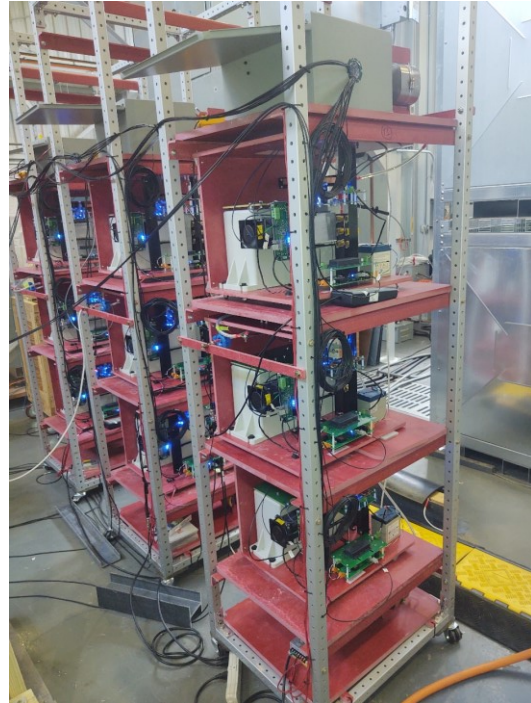
Florida State MMC converter 330kVA @ 4160V AC
