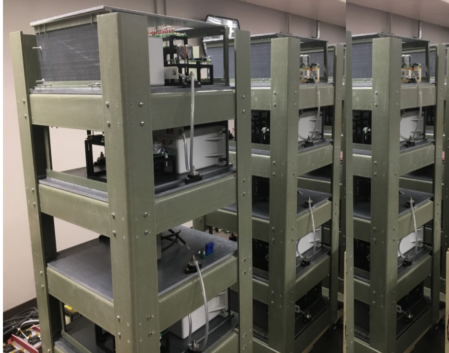
Ohio State MMC converter 330kVA @ 4160V AC
