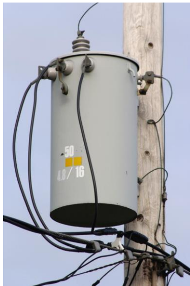
Traditional Pole-Mounted Transformer (No Power Electronics)
