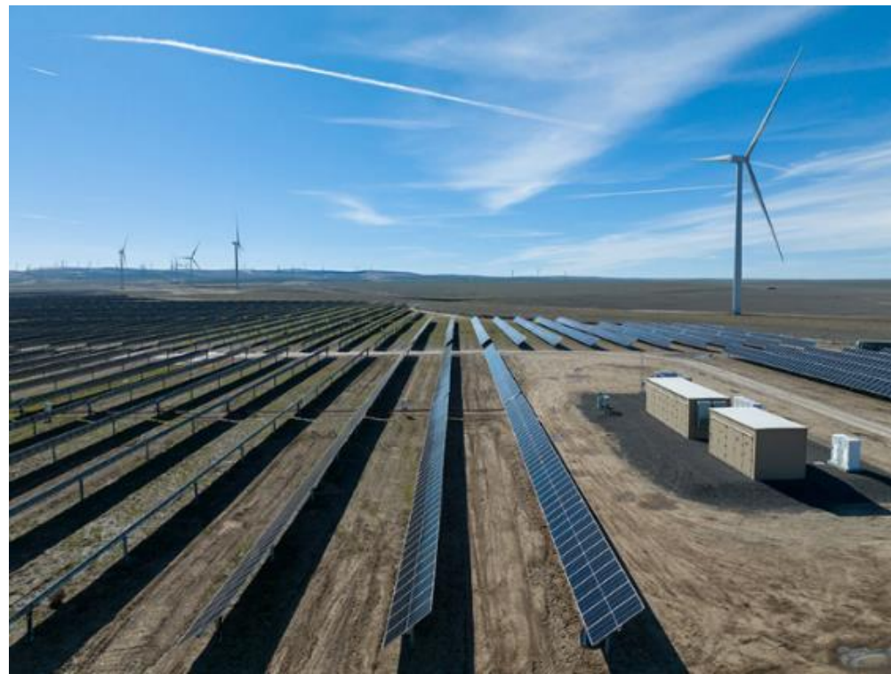
380MW Wheatridge wind, solar and battery storage power plant
