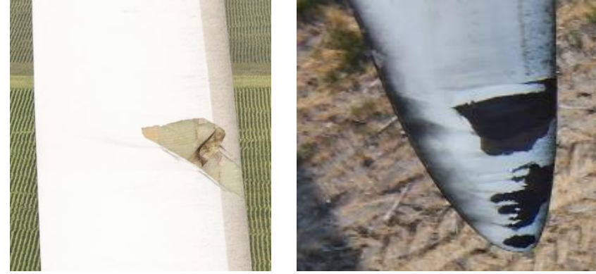
Chip Tip Damage
