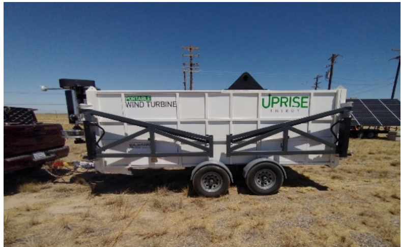
Figure 8. Uprise Energy system in trailer mode (photo from Idaho National Lab)
