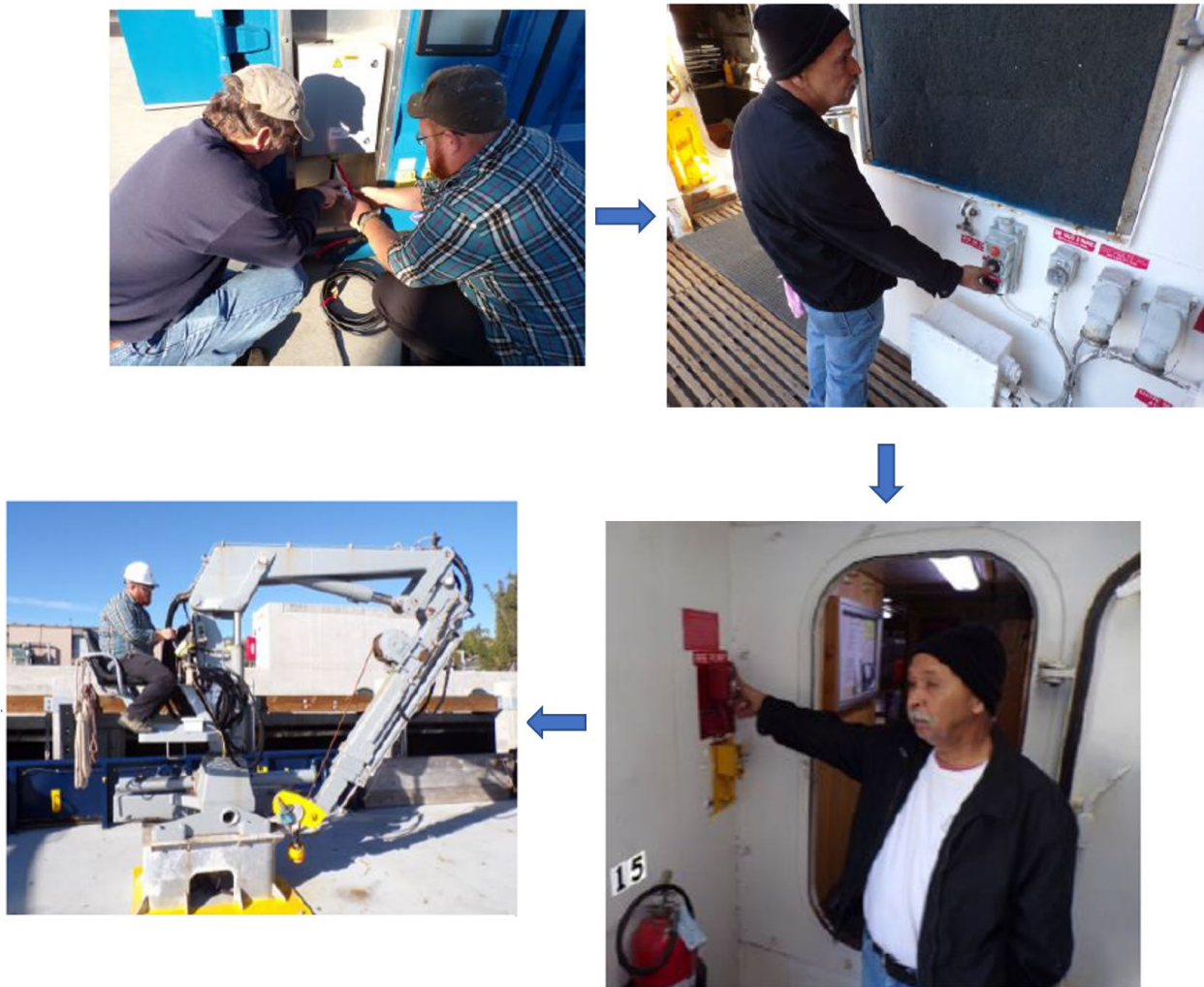
Figure 22. The initial powering of the R/V Robert Gordon Sproul mechanical systems with the MarFC on 12/19/19. Proceeding clockwise from the upper left, Captain Chris Welton (left) and James McManus connect the 480 VAC 3-phase vessel cable to the MarFC via the new junction box; Ernesto Bayer turns on a deck pump; Ernesto Bayer turns on the fire pump systems; and James McManus tests the operation of a deck crane while operating on MarFC power.
