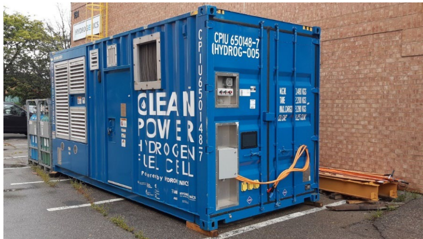
Figure 14. The 100-kW MarFC unit in place for electrical testing at Hydrogenics in FY 2019.
