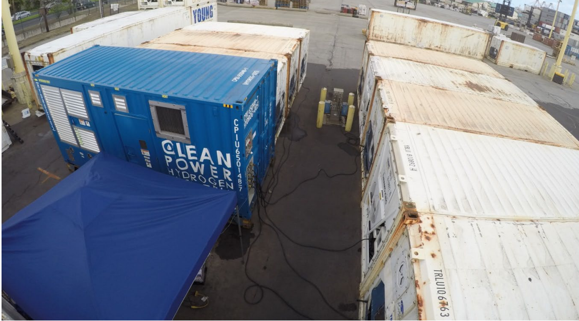
Figure 3. The blue MarFC unit providing power for reefers at the Young Brothers Ltd. facility in Honolulu, HI.
