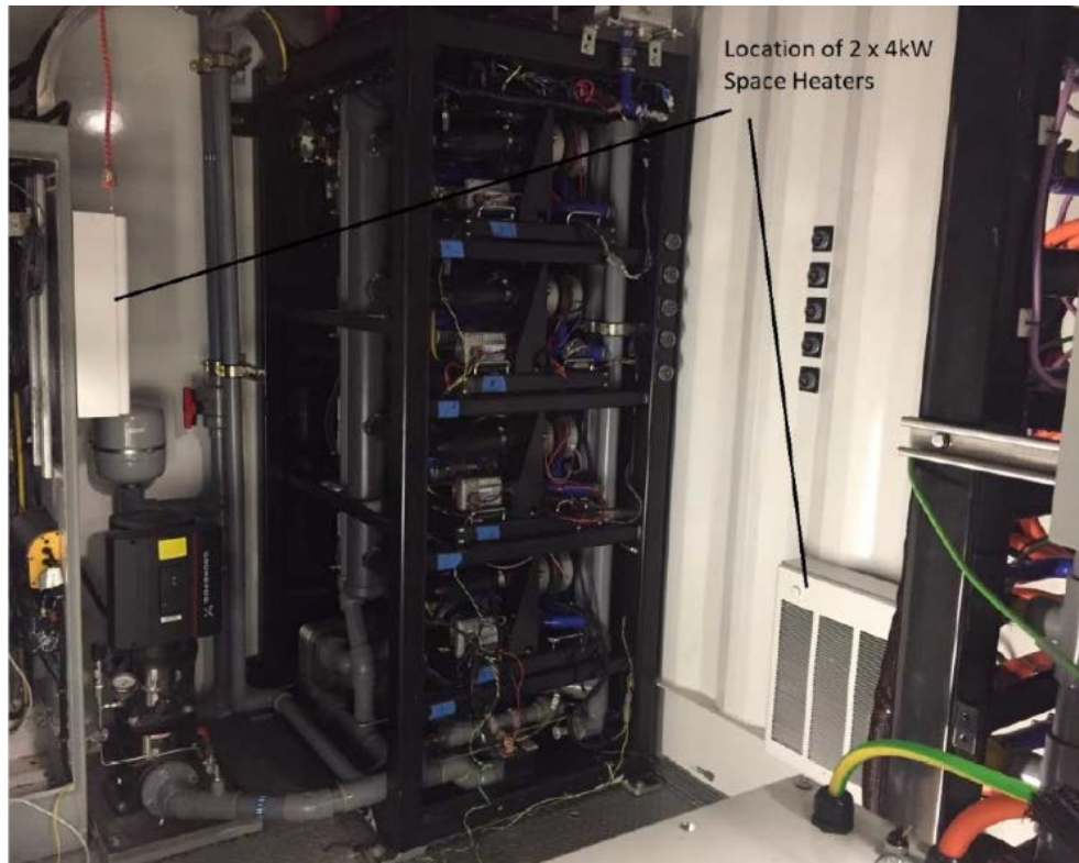
Figure 7. System heaters and controls that were installed to allow the MarFC to operate in weather down to -25°C in anticipation of a future deployment in cold weather.
