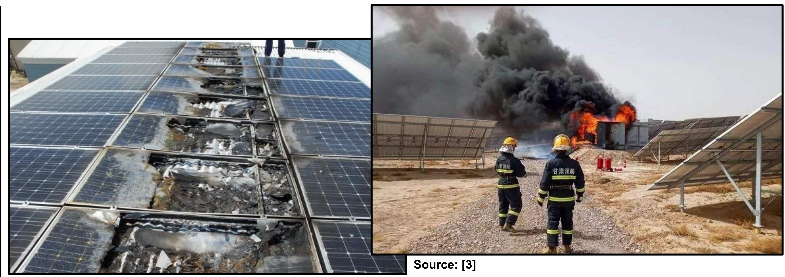
Fig. 1. Incidents showcasing examples of damage to solar PV modules and instance of fire in a solar station resulting from connector failures.
