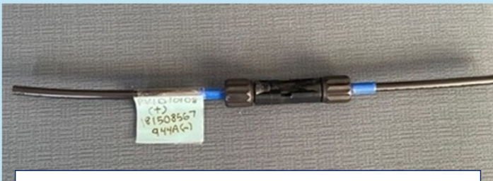
At least 10" of cable should remain at both ends; the connector itself should be left intact and labeled
