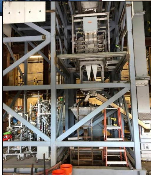
Integration of heat exchanger and sCO 2 flow loop in tower
