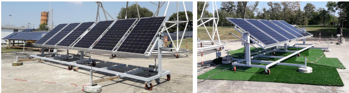
Figure 107: Bifacial PV system under test; South-facing PV module on light grey concrete tilted 30°(left); South-facing PV modules on synthetic green grass tilted 30° (right).
