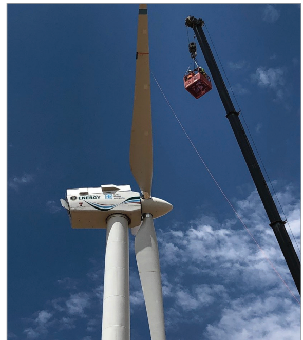
SWiFT site personnel with Sandia safety engineering inside manlift basket preparing to remove the lifting straps from the NRT rotor following installation onto SWiFT Turbine A1.
