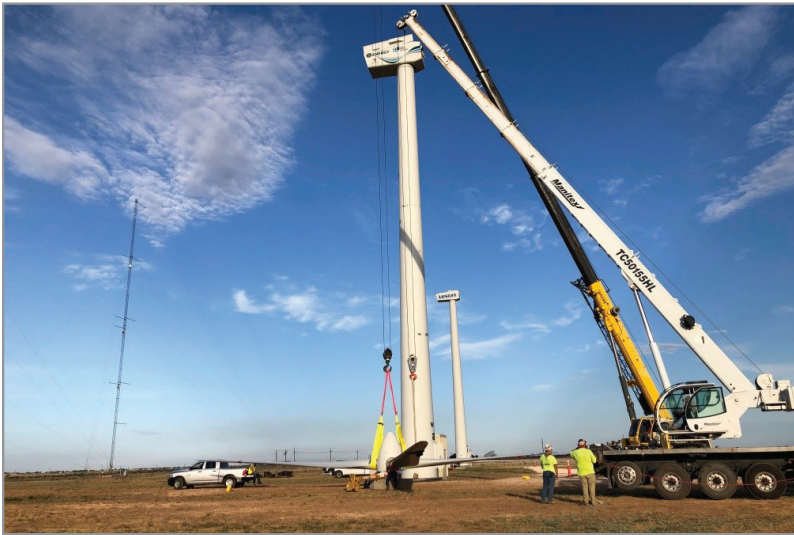
Lifting straps connected to the NRT rotor in preparation for the lift and installation onto SWiFT Turbine A1.
