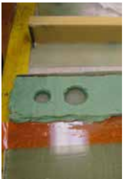
Voids in bond joint
