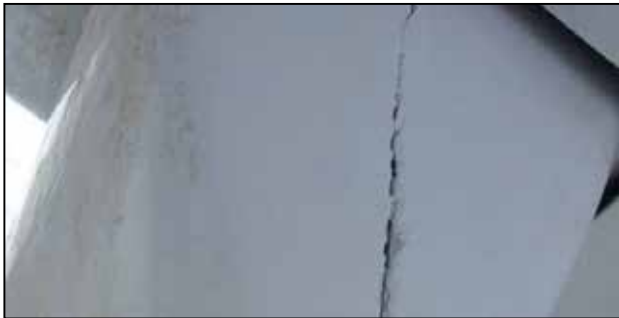
Severe Growth of Fiber Fracture
