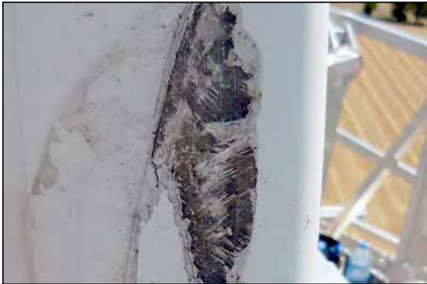
Lightning Strike Damage
