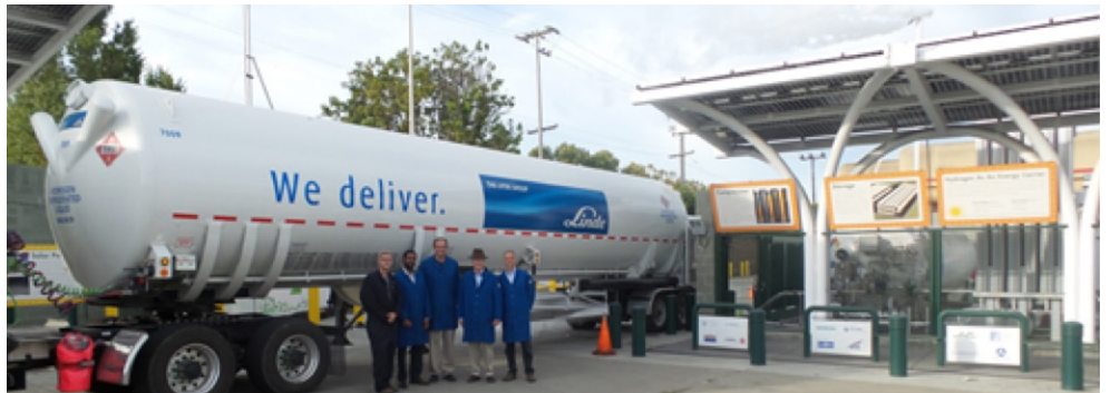
Figure 7: Examples of LH 2 tanks: (Top, Left) Chart Inc. LH 2 tank; (Top, Right) Linde Group LH 2 tank at the AC Transit Hydrogen Station in Emeryville CA and (Bottom) Linde LH 2 refueling trailer at the AC Transit Hydrogen Station
