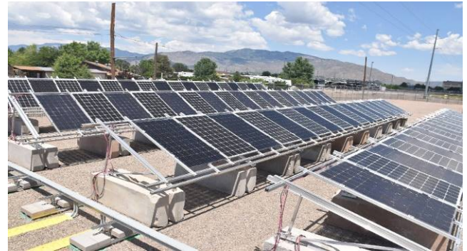
Fig. 9. Sandia's fixed-tilt string-level arrays, Albuquerque, NM.
