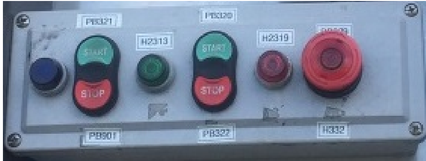
Figure 63: Slight fading of generator control buttons due to sun/UV exposure.
