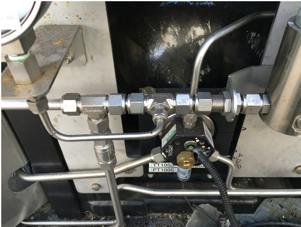
Figure 62: Some of the stainless steel piping inspected for corrosion after 9 months of deployment. Very little corrosion on the piping was observed.
