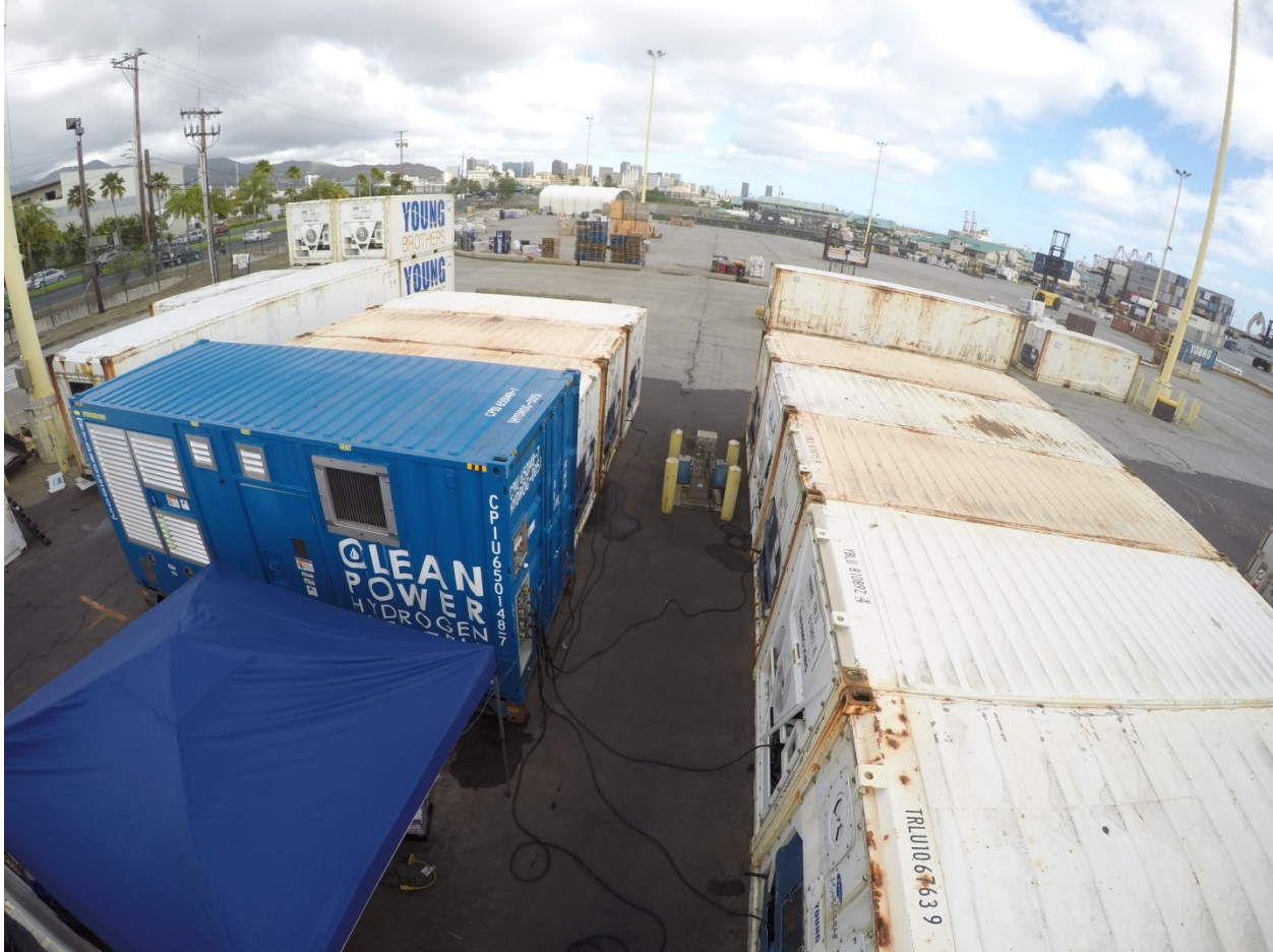
Figure 34: The generator (blue) in the Icehouse area powering reefers (white).
