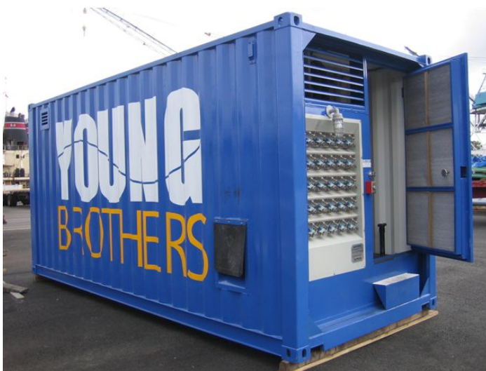
Traditional maritime diesel generator deployed at Port of Honolulu by Young Brothers, Ltd. Photo courtesy of Young Brothers, Ltd.
