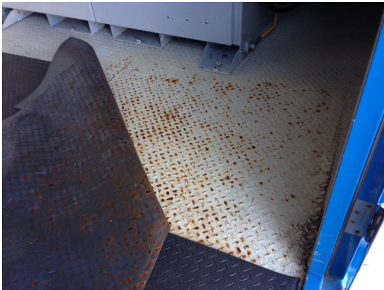
Figure 60: Generator room floor corrosion due to continual presence of mats. Mats were subsequently removed and the floor was re-painted with more robust paint.
