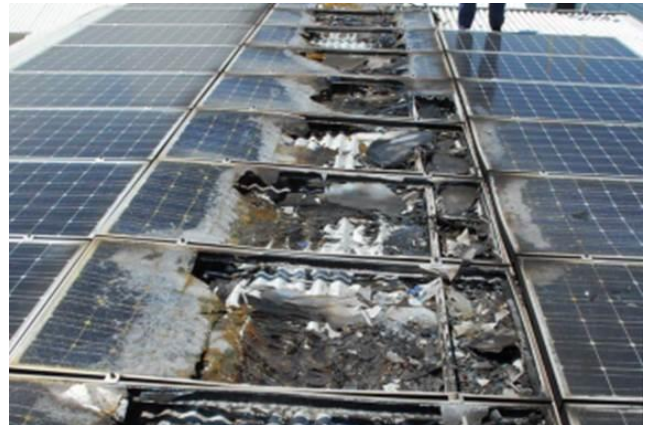
Fig. 1: Damage to a PV system attributed to an arc fault.
