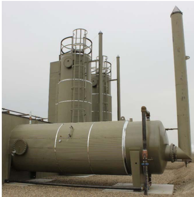
Figure 3-11. Installed Horizontal and Vertical HTs.
