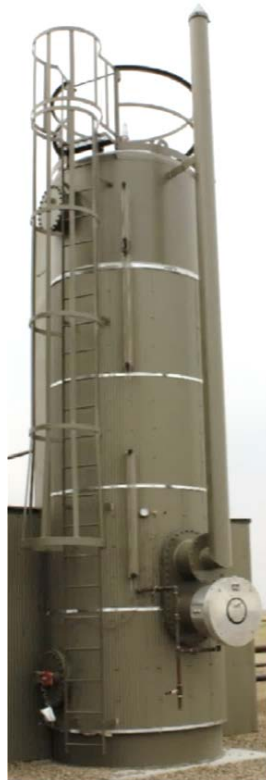
Figure 3-10. Installed Vertical HT.
