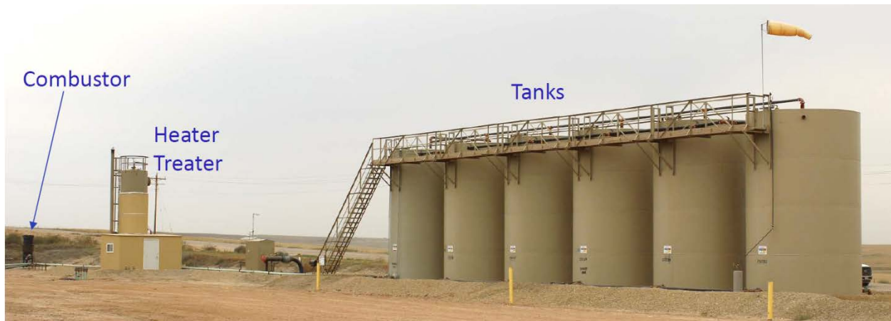
Figure 3-7. Bakken Well Site Conditioning Equipment Configuration.
