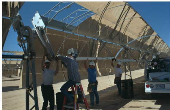
Figure 2 HCE freeze/thaw test rig in a 2-HCE configuration (top). The impedance heater electric connection can be seen at the top of the insulated standpipe. The standpipes approximate the expected orientation of the flex hoses during shutdown of a commercial plant (bottom), the time at which a freeze event is most likely. The HCEs are usually covered to prevent heatup due to one-sun exposure prior to first use (red cover on top, white cover on bottom).
