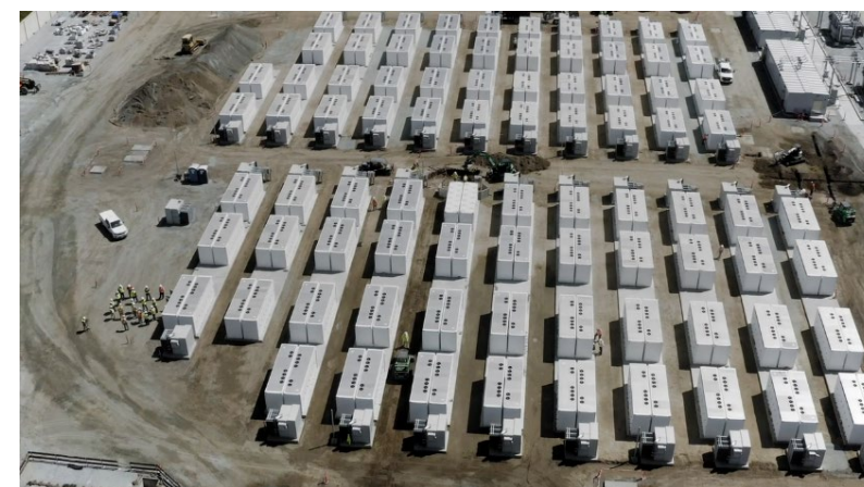
Tesla Megapacks, Moss Landing
