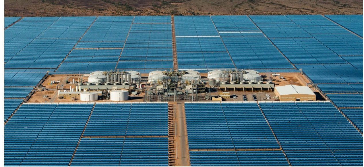
Solana Parabolic Trough Solar Project 1.5 GWh e storage in 6 pairs of hot and cold tanks.
