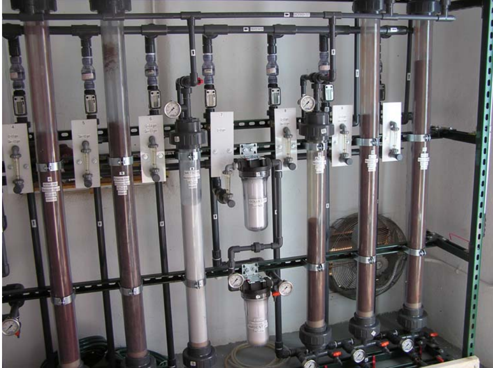
Figure 5. SNL Pilot Arsenic Treatment Pilot System. (Each of the four columns on left contains a different adsorbent medium. The 3 columns on right contain a single medium (AD33) with different contact times.)
