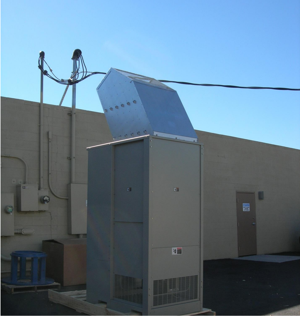
Figure 2-11. Avtron load banks.
