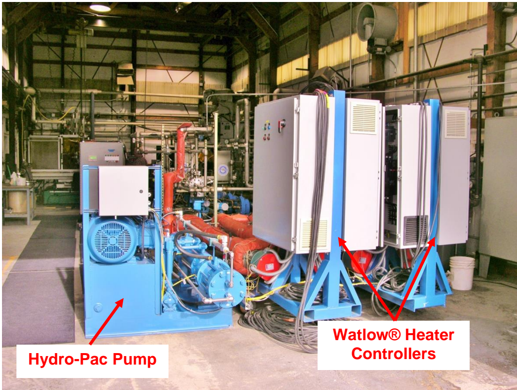
Figure 2-13. The new Hydro-Pac Scavenging Pump and Watlow® Heater Controllers.
