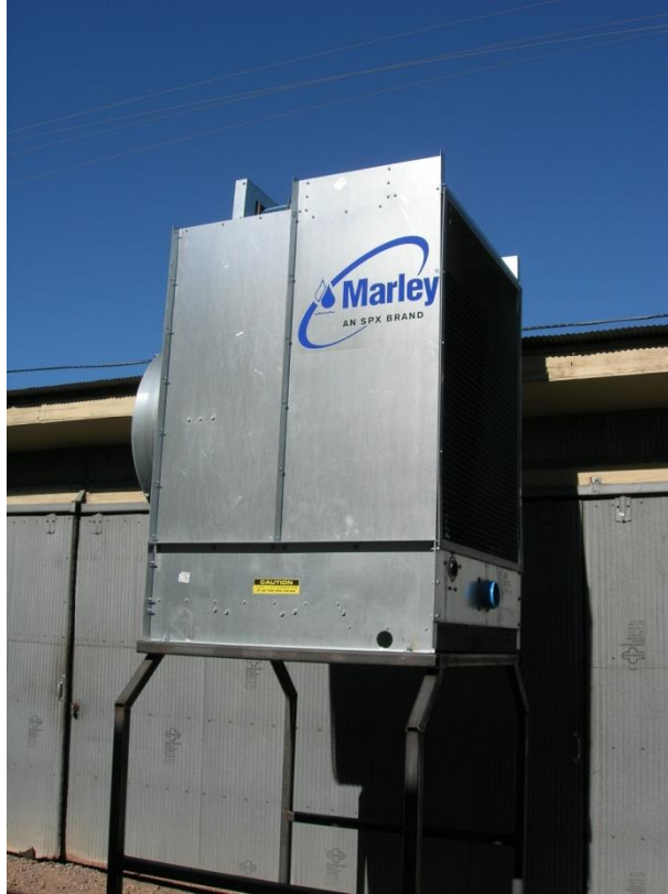
Figure 2-12. Evaporative Cooler. (The cooler has a name plate cooling capability of 220 kW.)
