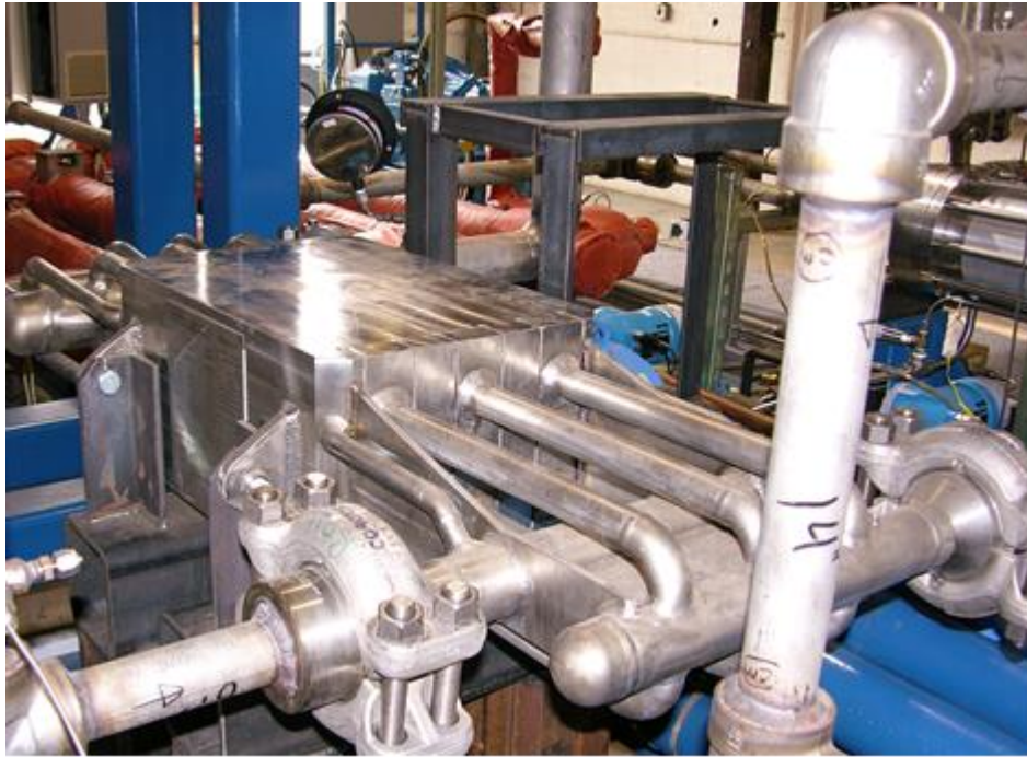
Figure 2-9. S-CO 2 LT PCHE recuperator.
