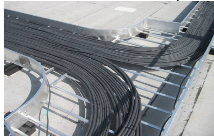
Modified - Cable Tray
