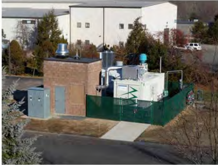
Figure 9: Fuel Cell Energy DFC300 MCFC power plant. Photo from Reference [44].
