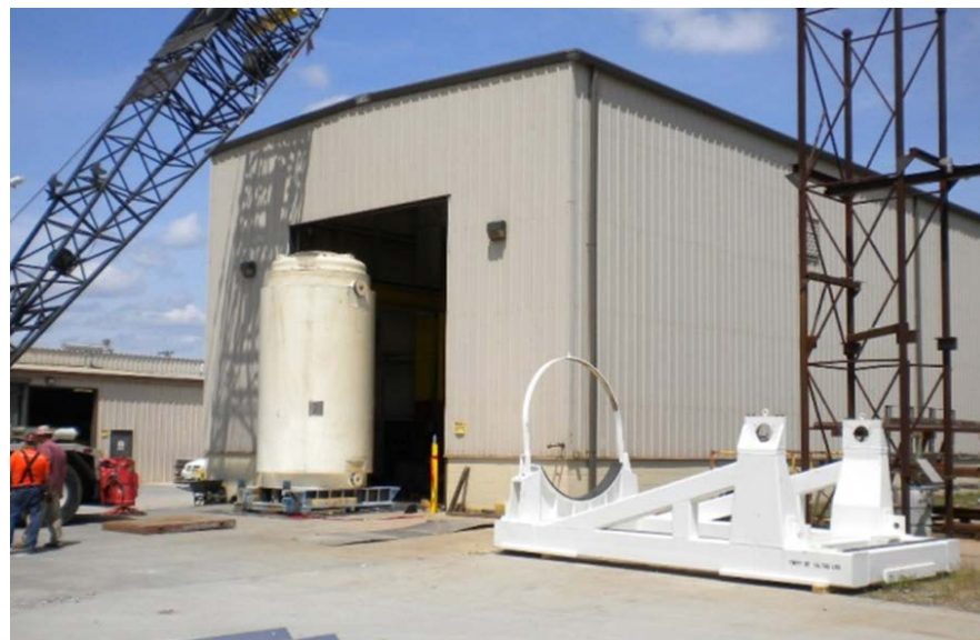
TN 32B cask being placed in Columbiana Hi Tech Building in Greensboro, NC
