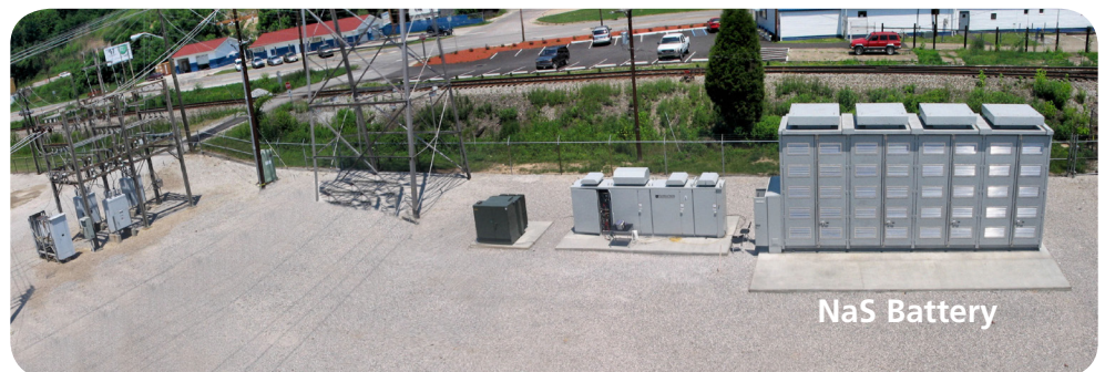
This Sandia-led DOE Office of Electricity demonstration project proved the effectiveness of sodium-sulfur batteries in peak shaving and capital deferment.
